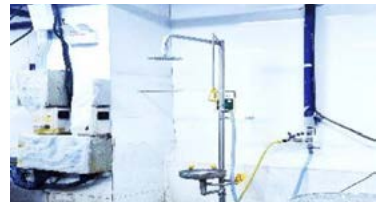
Emergency Shower Facilities
